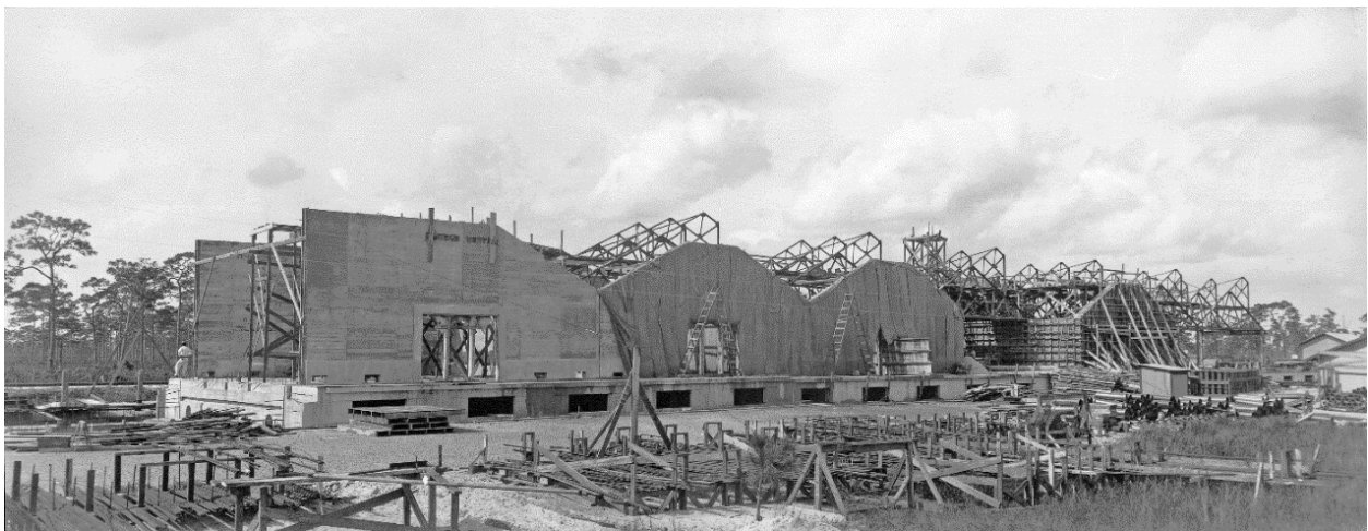
Photo 2: Red Hill storehouse construction, 1930. The steel girders and poured concrete used by project engineer Alexander Blair are visible here. Photo credit: Archbold Biological Station.
